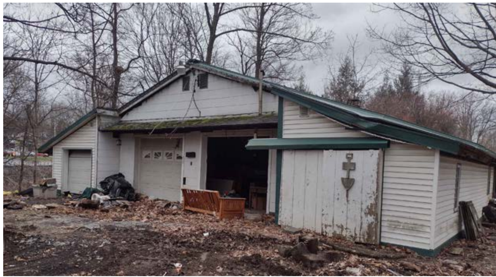
1 A100 VIEW OF GARAGE TO BE REMOVED & NEW RESIDENCE PROPOSED IN SAME LOCATION SCALE: N.T.S.
